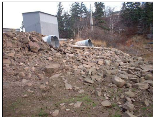
Figure 29. Upstream of crossing; two steel culverts placed high on the rock bank.
