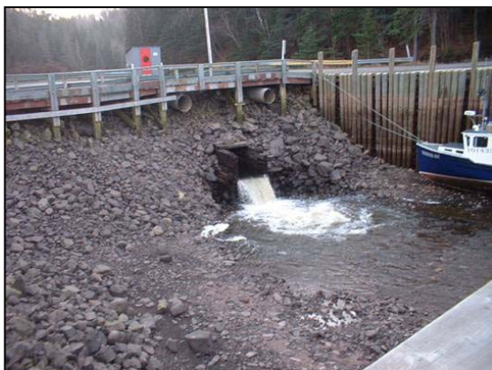
Figure 28. Downstream view of crossing showing outflow of freshwater into the harbour at low tide.
