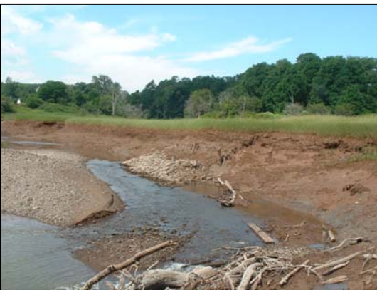
Figure 10. Collection of debris upstream of crossing.
