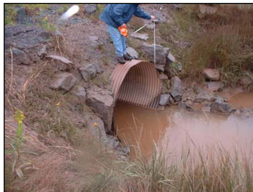
Figure 18. Culvert opening is smaller than stream width.
