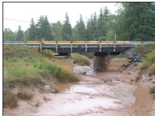
Figure 19. New wooden support structures have been built half way down the banks of the creek. The pinching of the creek by the support structures can be seen by looking at the high water line. (Photo taken downstream of the bridge.)
