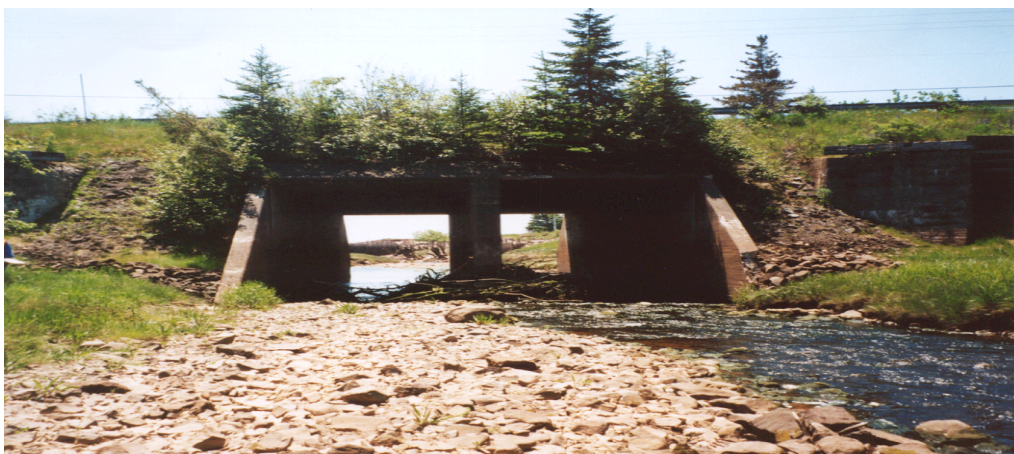
Figure 32. Upstream view of debris built up at site CBNS14C (Carrs Brook Road).
