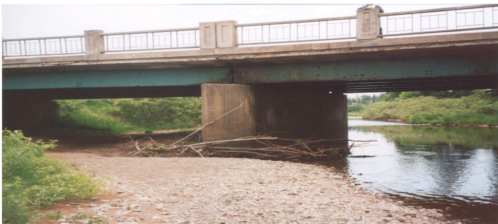
Figure 29. Upstream view of debris built up at site CBNS2B (Debert River).
