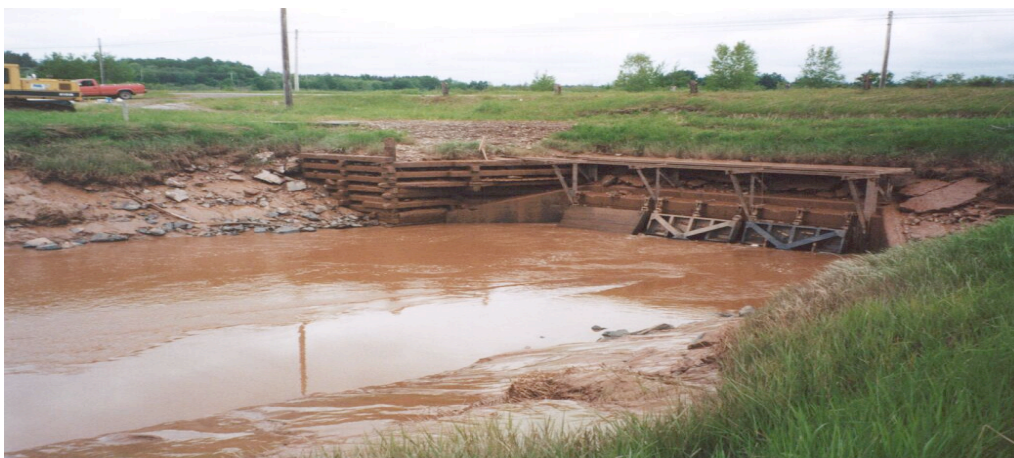
Figure 28. Downstream view of an aboiteau system with three tide gates at site CBNS1A (Chiganois River).
