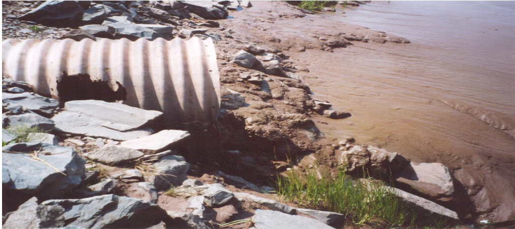
Figure 24. Downstream view of a corrugated steel culvert at site CBSS8C (Cobequid Trail).
