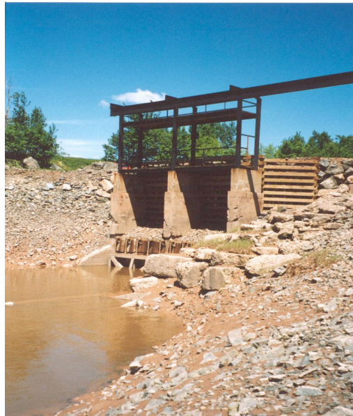
Figure 30. Downstream view of a large aboiteau at site CBNS5A (Great Village River).
