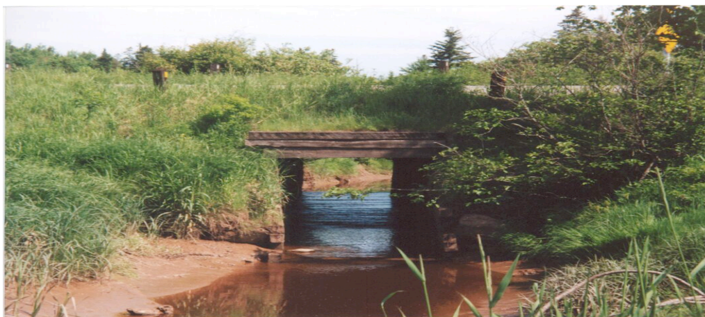
Figure 27. Downstream view of a wooden box culvert at site ST7C (MacKay Siding Road).
