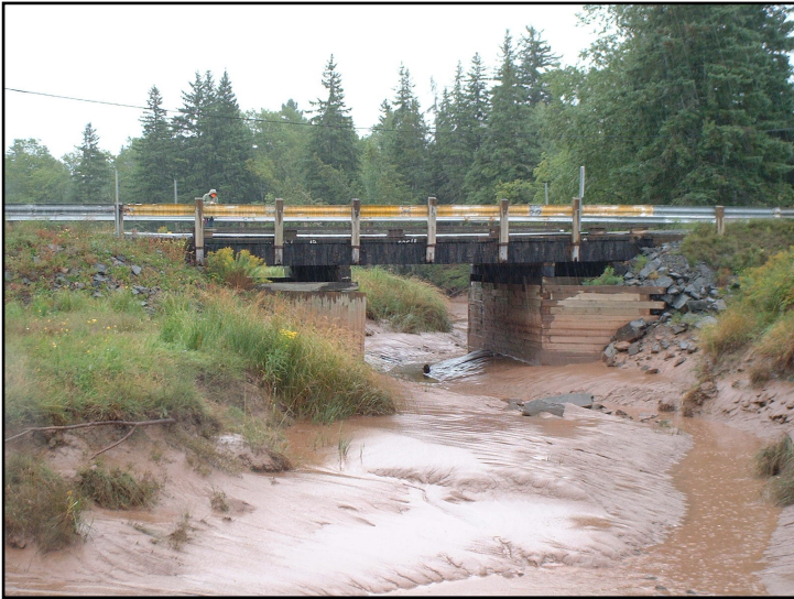
Figure 1: New wooden support structures have been built half way down the banks of the creek. The pinching of the creek by the support structures can be seen by looking at the high water line. Photo taken downstream of the bridge.
