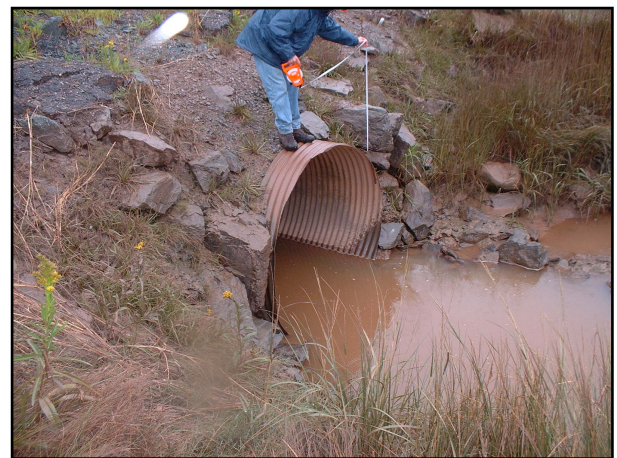
Figure 1: This photo shows the creek being wider than the culvert.
