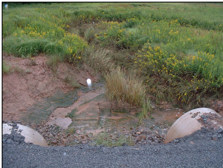
Figure 2: Downstream end of culverts showing a divergent channel, evidence of recent work and a new shoulder.
