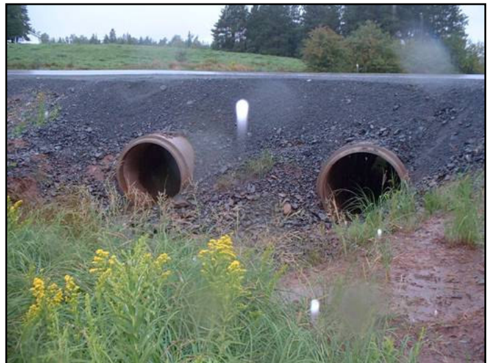
Figure 1: Downstream showing that the culverts are placed above the base of the channel. The background shows a definite elevation rise and a mix of agriculture and woodland upstream.
