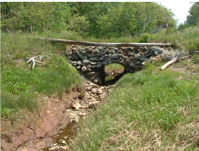
Figure 3. Remnants of old bridge downstream of crossing causing some further restriction
