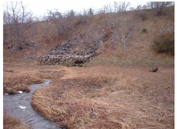
Figure 4. Downstream view of crossing DC6C, completely obstructed by rock.
