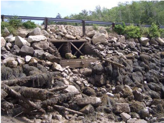
Figure 1. Downstream view of crossing. Culvert is filled with debris and placed high above creek bottom with large amount of rock and wooden debris.
