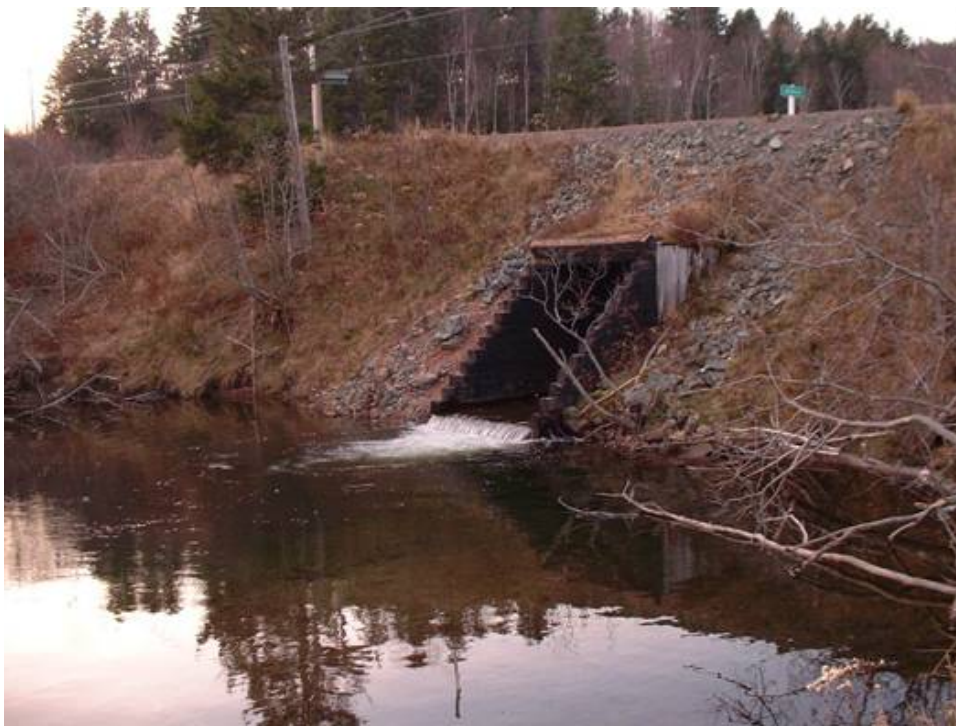
Figure 1. Downstream of crossing. The large pool in front of the culvert is visible as well as the high placement of the culvert.
