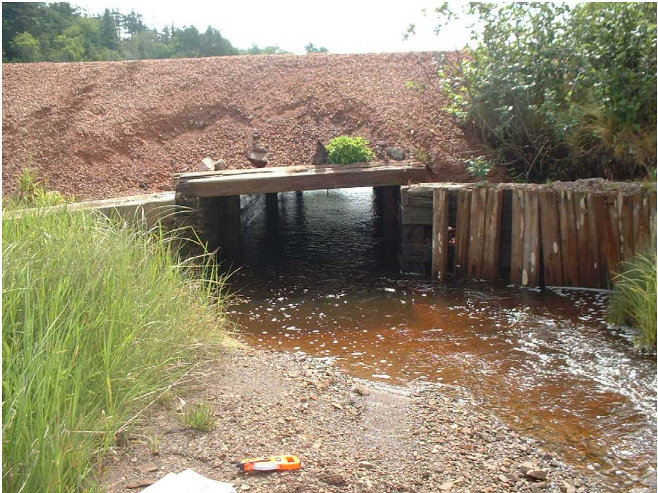
Figure 2. Upstream view of the culvert showing that the culvert is placed slightly off to one side with some pooling and slack water occurring to the sides of the culvert.
