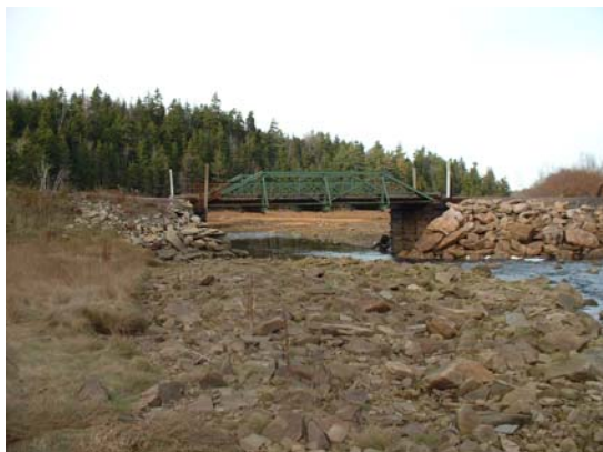
Figure 1. Downstream of the bridge clearly showing the build up of the banks with boulders.
