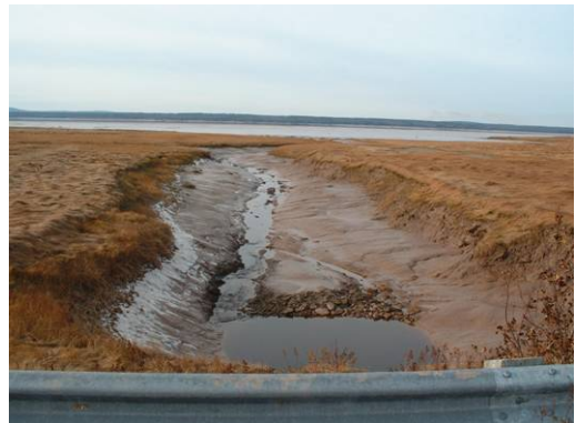
Figure 4. Downstream creek from the road. The pooling is evident in this photo.
