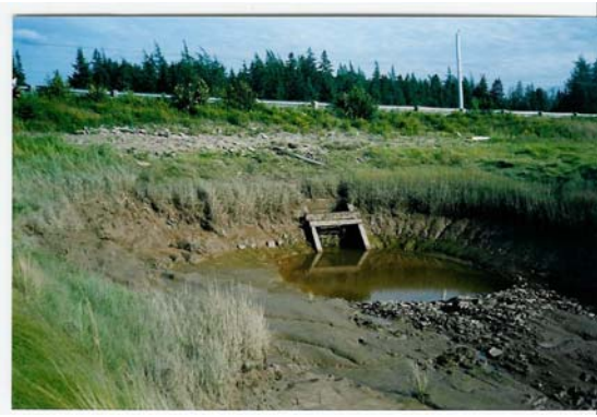
Figure 1. The downstream view of the culvert showing the bank erosion from pooling and perspective on how small the culvert is with respect to the pool.
