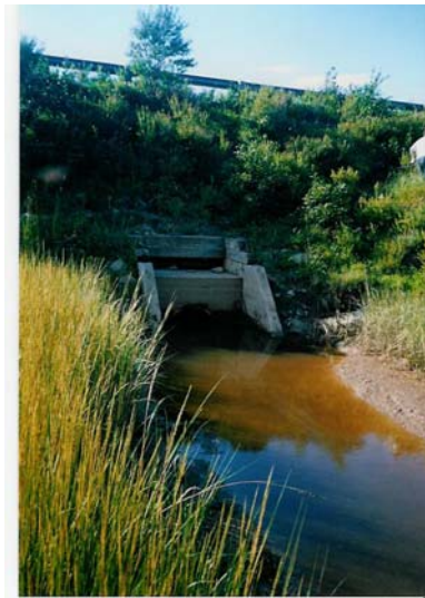
Figure 3. Upstream side of the culvert. There is a slight pooling in front of it. The old wooden box culvert is easily visible, with just the top of the round concrete culvert visible.
