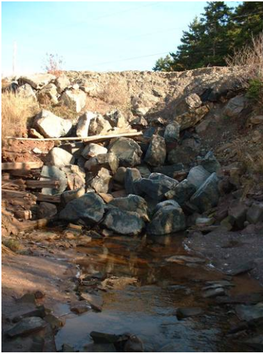
Figure 1. Downstream end of crossing completely buried by rock and other materials. Unclear as to whether a tidal gate is present or not. Damage to shoulder of road surface evident in picture.
