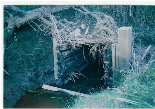
Figure 3. The upstream side of the culvert. Some debris is visible as well as damage to culvert.
