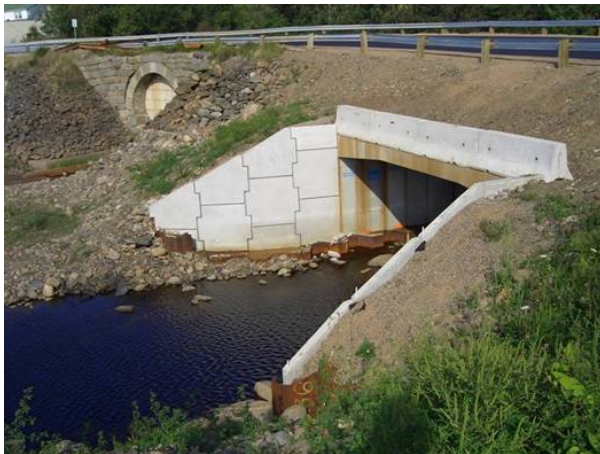
Figure 1. Downstream view of crossing, old sealed crossing to the left of new culvert
