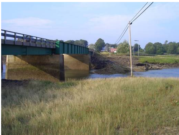
Figure 1. Upstream view of bridge showing large rock pile near base of bridge.
